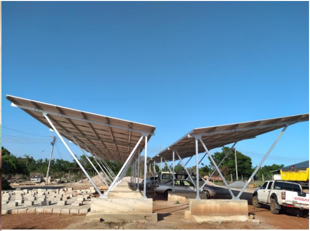
Power System Plant, will serve as car park
